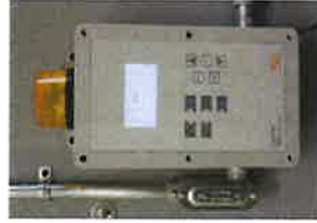
Cooler Control Panel
