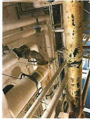
Rotting Pipe at Riley Elementary
