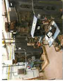
Leighton Elementary Boilers
