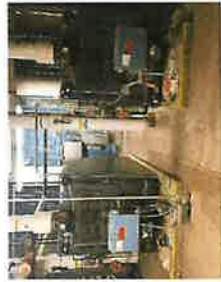
Riley Elementary Boilers
